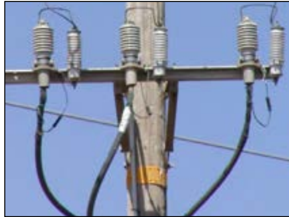
Figure 5-85. Three-phase grounded metal bracket with uncovered potheads, arresters, and stinger wires.
