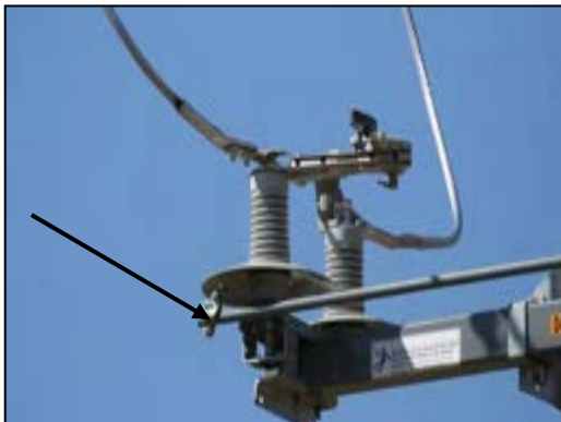
Figure 5-80. Switch with barrier plate.
