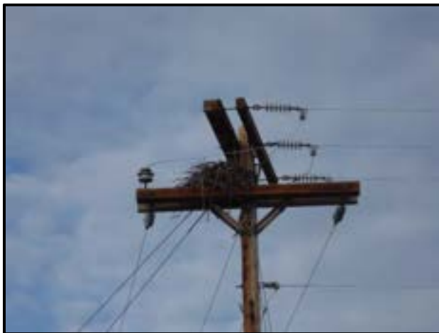
Figure 9-1. Problem Red-tailed Hawk nest on an unprotected distribution line.
