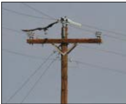
Figure 5-10. A typical ridge-pinned tangent structure retrofitted with conductor covers (Power Line Sentry, LLC).
