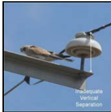
Figure 6-13. Lesser Kestrel perched on a grounded steel distribution crossarm.
