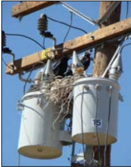
Figure 2-23. Common Raven nest on a transformer bank.
