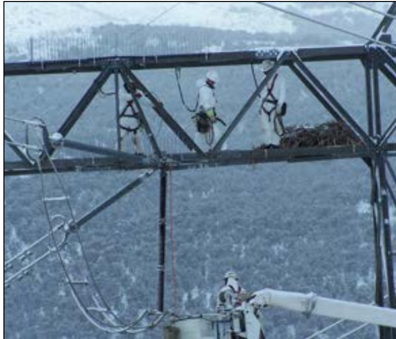
Figure 10-4. Raptor Guard Spike Perching Excluders being installed to prevent perching and defecation on transmission insulators (Power Line Sentry, LLC).
