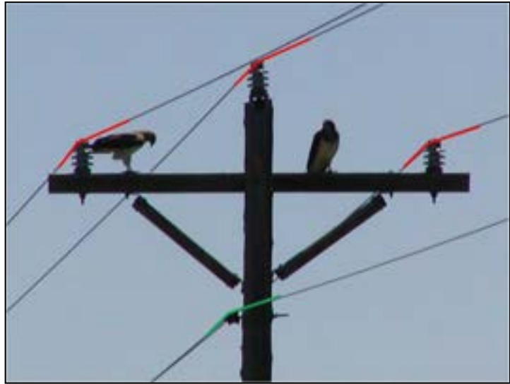
Figure 2-5. Hawk-friendly pole has adequate separation between energized (red) and grounded (green) components.
