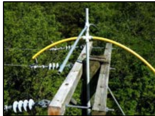
Figure 9-13. Stick deflector restricts the area to build a nest and flexible tubing makes an unsteady perch (Power Supply Company)
