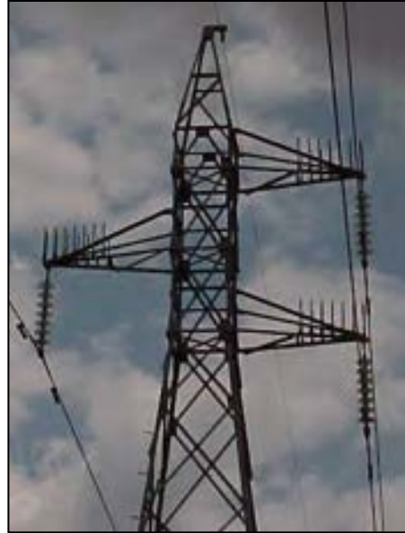
Figure 10-2. HDPE spikes deployed on the arms of a lattice transmission structure (Mission Engineering).
