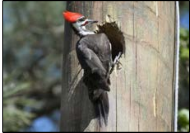
Figure 9-20. Pileated Woodpecker and nest cavity in a wood pole.
