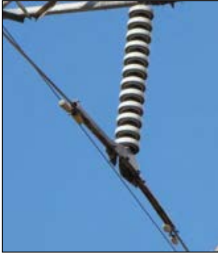
Figure 10-7. Conductor cover on center phase (TE Connectivity).
