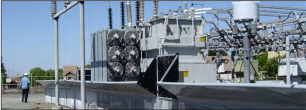
Figure 7-19. Kinectrics PowerKage (Kinectrics).
