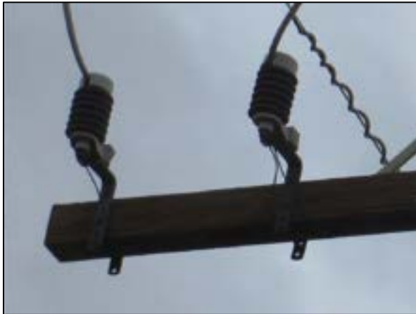
Figure 5-62. Bare arrester grounds are shielded from avian contact by the crossarm.
