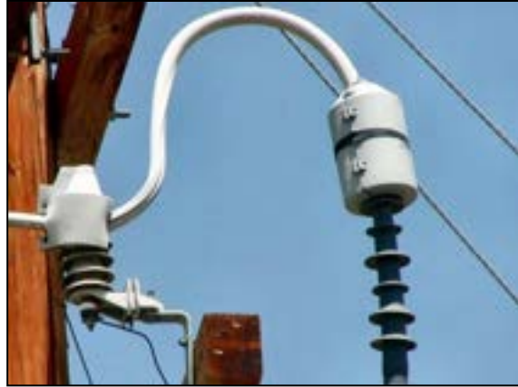
Figure 5-69. Protected riser pole (Hubbell Power Systems, Inc.).
