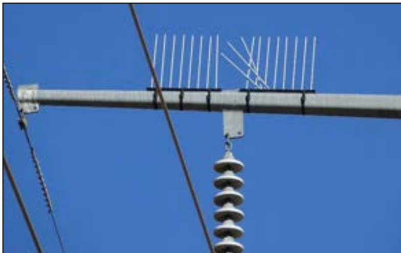
Figure 10-3. Raptor Guard Spike Perching Excluders with angled spikes to block perching above insulators (Power Line Sentry, LLC).
