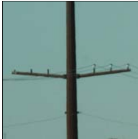
Figure 6-15. Steel distribution underbuild crossarms with inadequate horizontal phase-to-phase separation, plus inadequate horizontal and vertical phase-to-ground separation.
