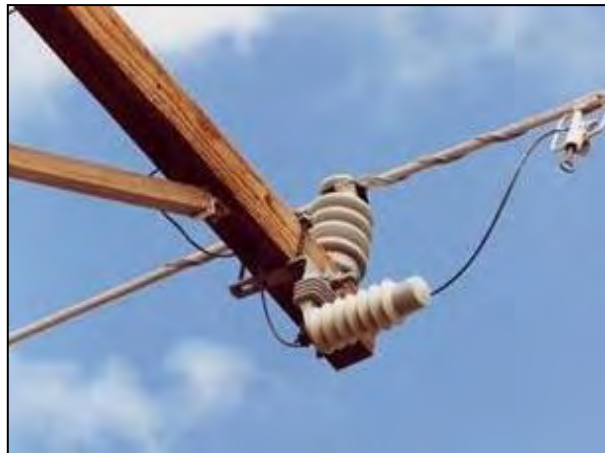
Figure 5-61. Underarm horizontally mounted surge arrester reduces animal exposure.
