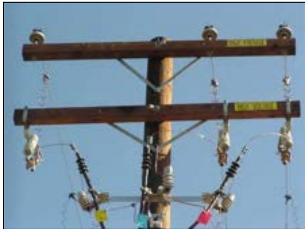
Figure 5-65. Unprotected potheads on a riser pole.
