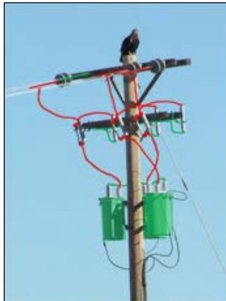
Figure 2-4. Complex transformer pole with many jumper wires, and little separation between energized (red) and grounded (green) contacts.
