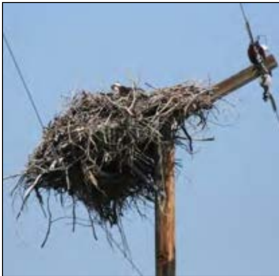
Figure 2-21. Osprey nest affecting the viability of a wood distribution structure.
