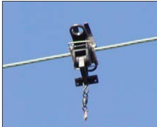
Figure 8-20. Broken hardware on active line marker
