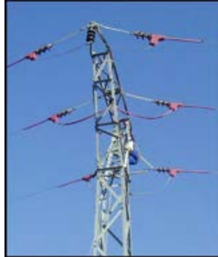
Figure 10-8. Jumper cover for double deadend transmission structure (TE Connectivity).
