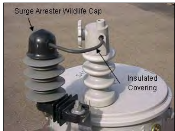
Figure 5-57. Transformer mounted surge arrester with wildlife cap.
