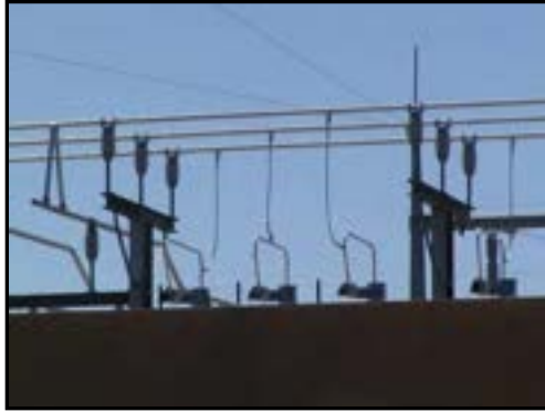
Figure 7-2. Substation bus supports for animal protection.
