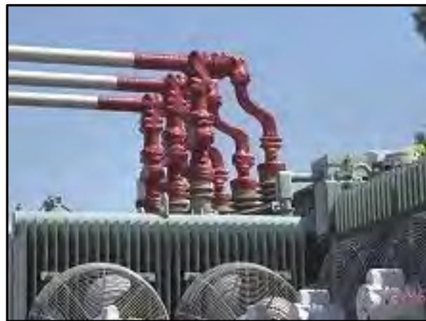
Figure 7-1. Insulating materials applied to substation bushings and busswork.
