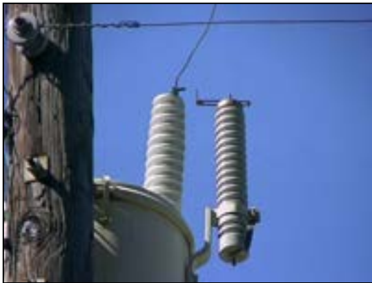
Figure 5-58. Transformer with gapped arrester.
