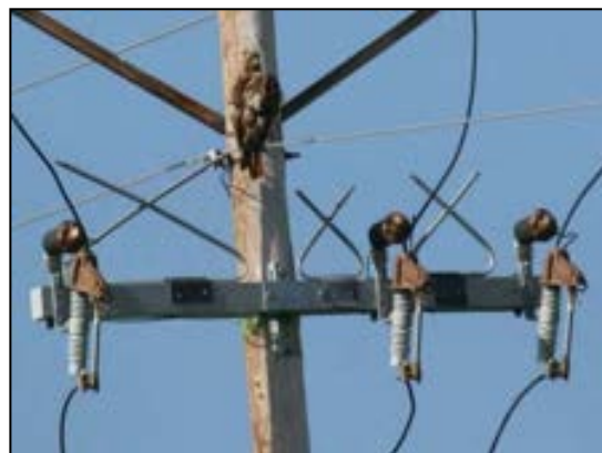
Figure 5-87. Three-phase fiberglass arm with covered cutouts, arresters, and stinger wires. Perch discouragers provide redundant protection.
