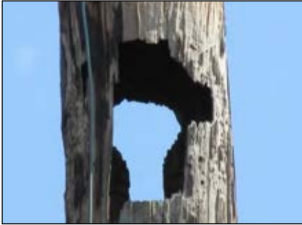
Figure 2-25. Severe damage resulting from Pileated Woodpecker nesting or roosting cavity (Ron Pope).
