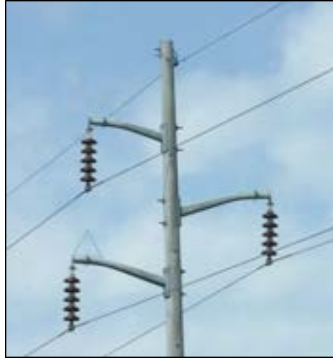
Figure 10-10. Perch discouragers designed to shift large birds away from the insulators.
