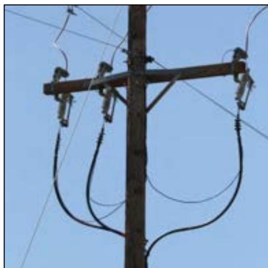
Figure 5-72. Potheads suspended from cutouts.
