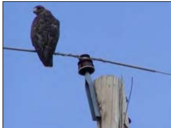
Figure 5-83. Exposed pole-top ground wire
