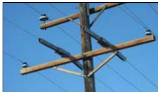
Figure 5-11. A typical flat-top tangent structure retrofitted with conductor covers (Eco Electrical Systems).
