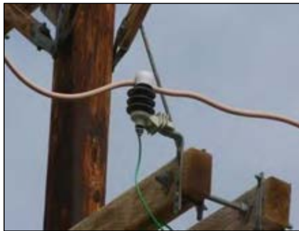
Figure 5-64. Surge arrester with cap and insulated ground wire.
