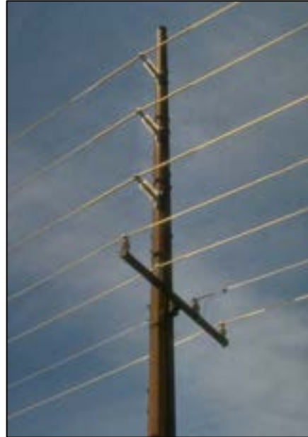
Figure 6-4. Hazardous vertical configuration with metal pole grounding line post insulator bases.
