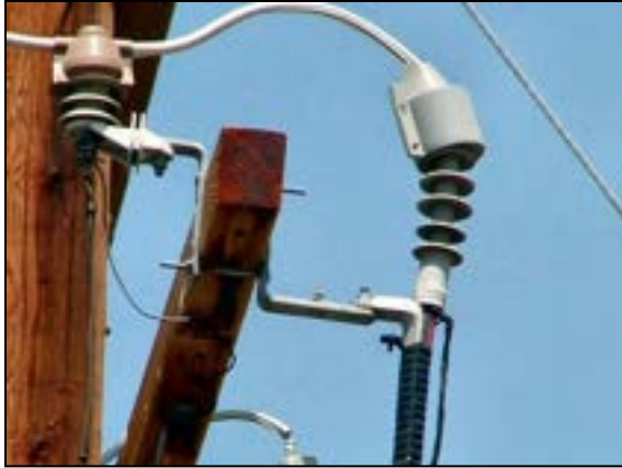
Figure 5-68. Protected riser pole (Salisbury by Honeywell).
