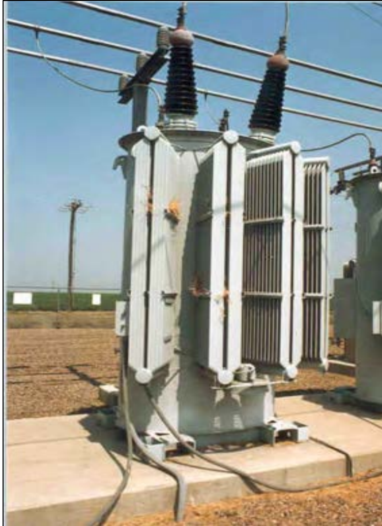
Figure 2-9. Nests in substation transformer cooling fins (EPRI).
