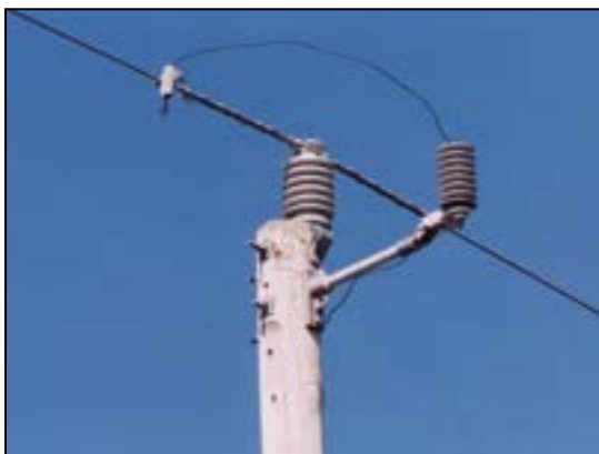
Figure 5-86. Single-phase ungrounded fiberglass bracket.
