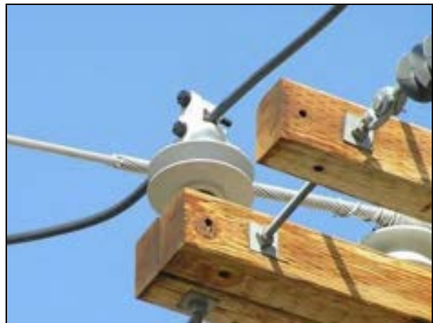
Figure 5-38. Covered jumper supported with a vice-top insulator (Hendrix).
