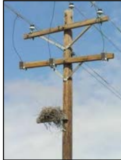
Figure 9-8. Raven platform below crossarms.
