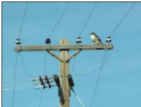
Figure 5-7. Flat-top unit does not provide adequate separation for hawks.
