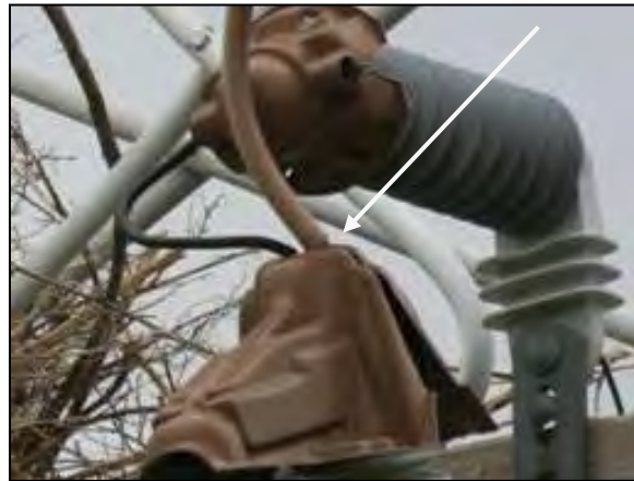
Figure 5-36. Cutout cover with gap between top of cover and bottom of stinger insulation.
