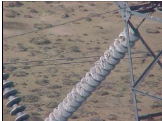
Figure 2-29. Accumulated avian excrement (bird pollution) on an insulator (Arizona Public Service).
