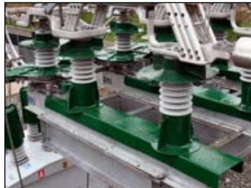
Figure 5-81. Switch with custom-formed barrier plates.
