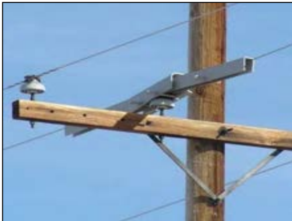
Figure 5-12. Eco Electrical Systems conductor cover.
