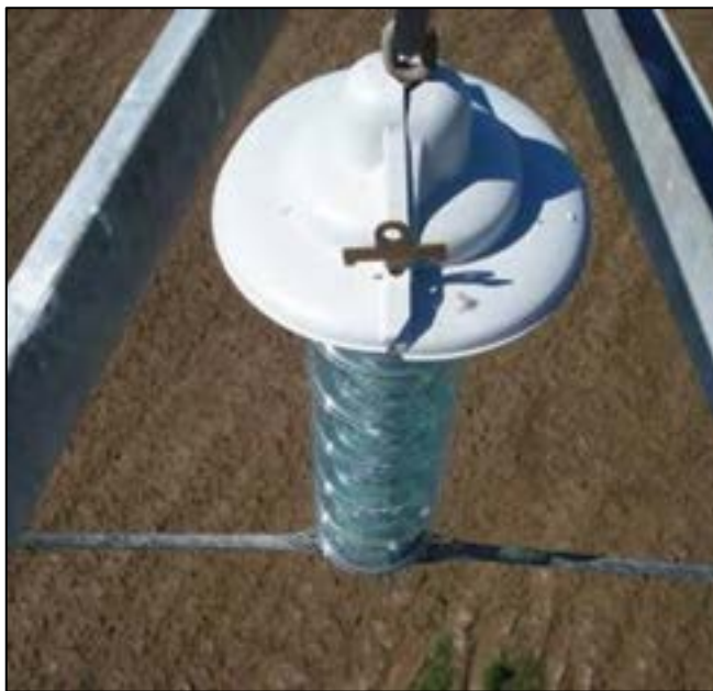
Figure 10-14. Bell insulator stream shield (Kaddas).
