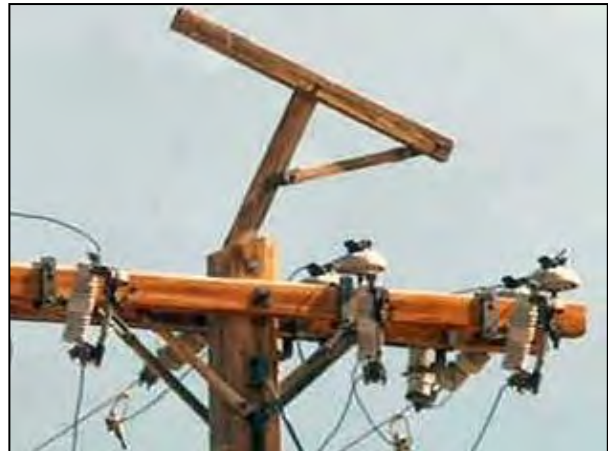
Figure 5-99. Improperly installed elevated perch and unprotected pole.
