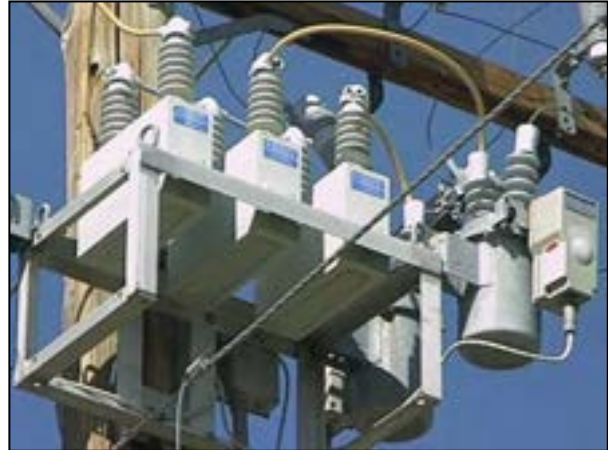
Figure 5-74. Capacitor bank factory-equipped with animal protection.
