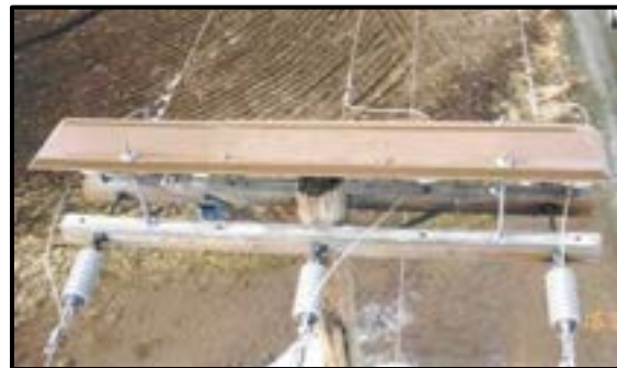
Figure 9-17. Stick deflector specifically designed to prevent nesting above the center phase on an H-frame structure (Kaddas Enterprises, Inc.).
