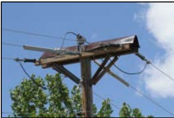
Figure 9-12. Stick deflector prevents nesting materials from being anchored between double crossarms (Power Line Sentry, LLC)
