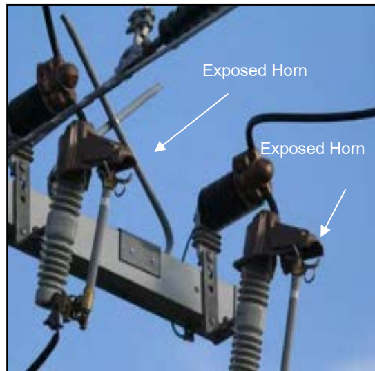
Figure 5-54. Protected cutout/arrester combination with exposed horns on the cutouts.
