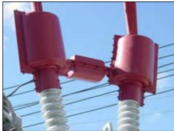
Figure 5-76. Regulator with bypass arrester cover (TE Connectivity).
