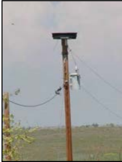
Figure 9-4. Nesting platform above a retrofitted single-phase pole.
