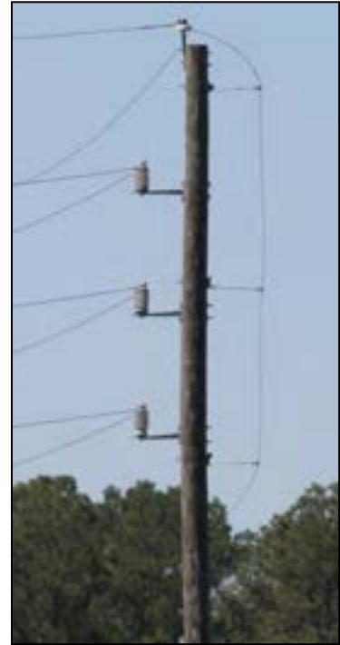
Figure 6-9. Ground wire routed to isolate from conductors.
