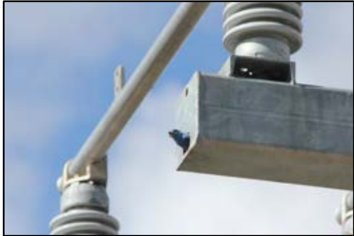
Figure 9-23. Bluebird nest in substation support arm.
