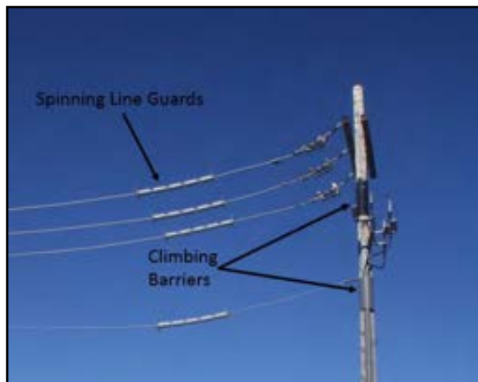
Figure 7-21. Substation getaway pole fitted with spinning line guard and climbing barriers.
