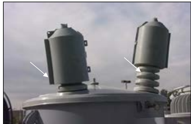
Figure 5-44. Hubbell Power Systems, Inc. bushing covers installed incorrectly (left) and correctly (right).
