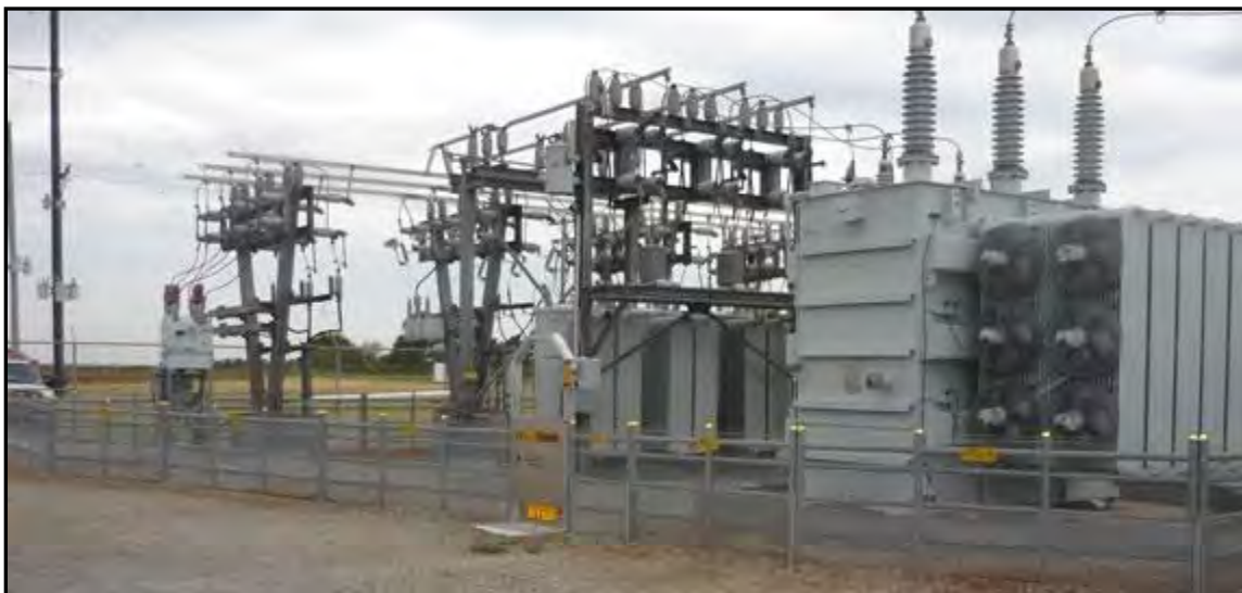
Figure 7-20. TransGard Systems, Inc. fence (TransGard Systems, Inc.).
