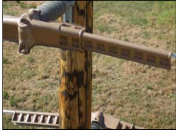
Figure 5-21. Bonded insulator bases mean each phase requires a conductor cover (Kaddas).
