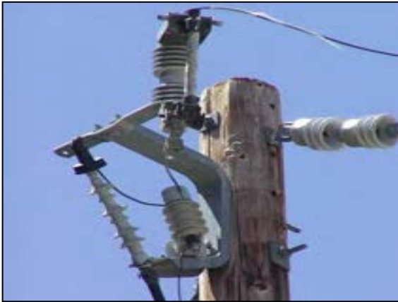
Figure 5-84. Single-phase grounded metal bracket with uncovered cutout, pothead, and stinger wires.
