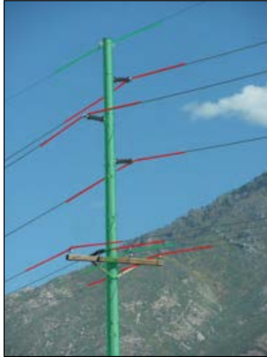
Figure 2-7. Steel transmission structure with little separation between energized (red) and grounded (green) contacts.
