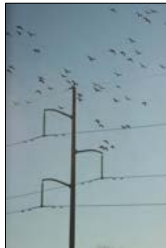
Figure 6-2. Vertical davit arm tangent structure is safe for perching birds.
