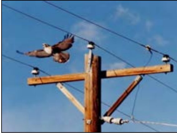
Figure 5-5. Typical tangent structure provides adequate separation for hawks.
