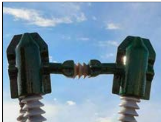
Figure 5-77. Regulator with bypass arrester cover. (Photo credit: Cantega)
