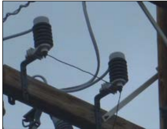
Figure 5-63. Bare arrester ground is exposed to casual avian contact.
