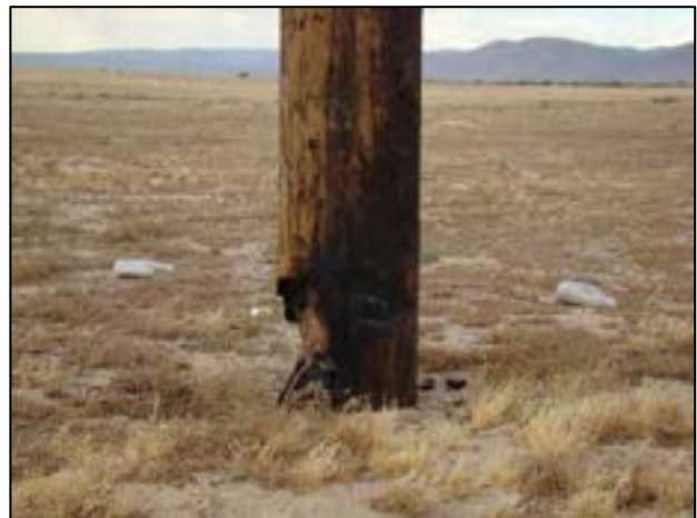
Figure 13-2. Compromised pole discovered during an ARA.
