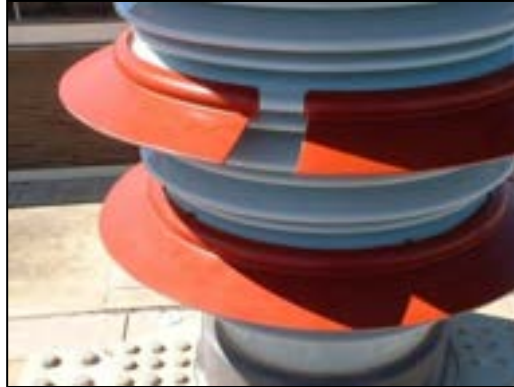
Figure 6-10. Creepage extenders (shown here in a traditional substation application) can also be deployed as barriers on line post insulators.
