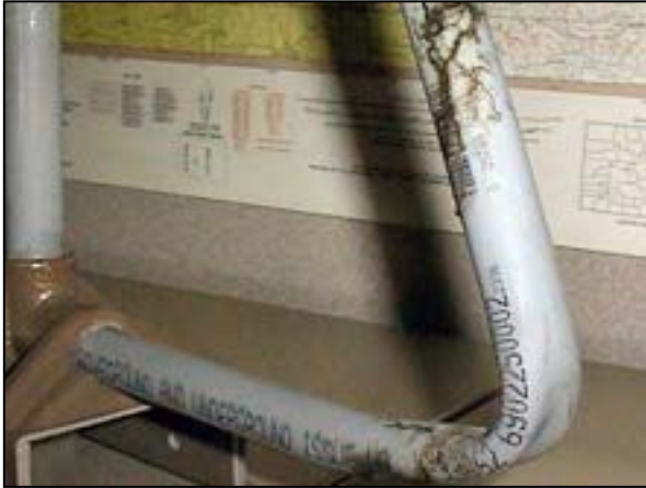
Figure 5-108. Flash marks on discourager.
