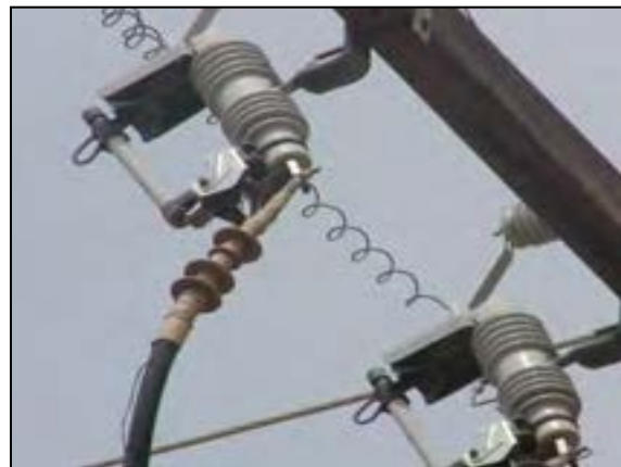
Figure 5-71. Pothead mounted below cutout.
