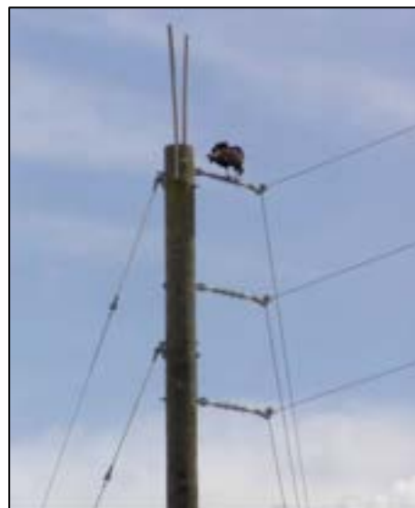
Figure 5-32. Avian-friendly three-phase vertical tangent structure with insulating links in guy wires.
