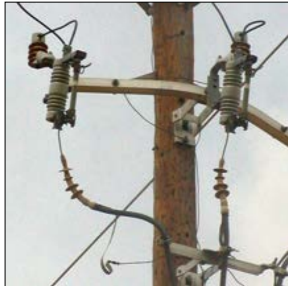
Figure 5-66. Unprotected potheads on a riser pole.
