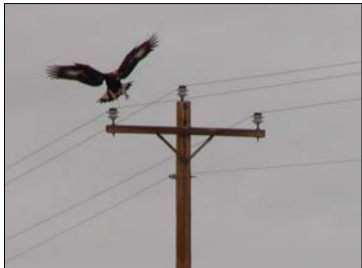
Figure 2-2. Example of Golden Eagle wing span relative to clearances between phase wires on a typical three-phase distribution structure.
