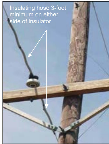
Figure 5-16. Conductor cover with additional insulating hose.
