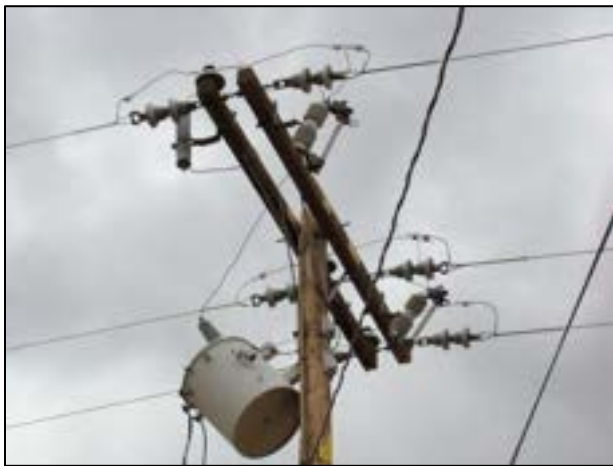
Figure 13-1. Failing transformer mount discovered during an ARA.
