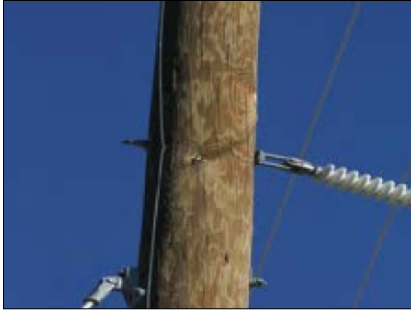
Figure 5-20. Ground wire routed away from hardware and conductors.
