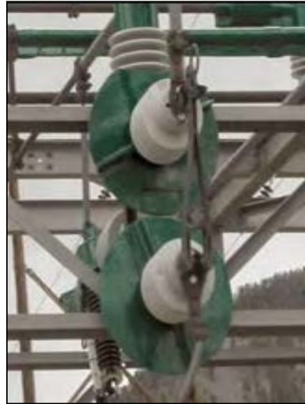
Figure 5-79. Barrier plate on switch (Cantega).
