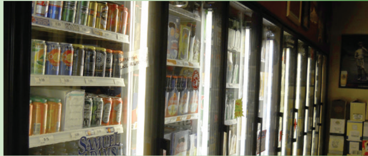
The reach-in coolers were retrofitted with new EC motors for fans, along with a two stage motor control that shifts fans to half speed when not in a cooling phase.
