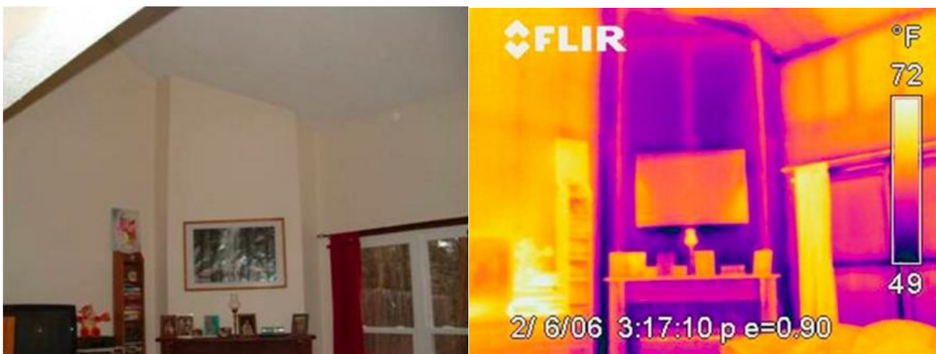
Infrared view of missing insulation
